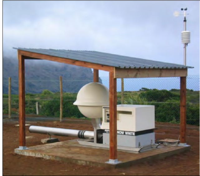
FIGURE 7. A Snow White HVAS situated at RN67.
